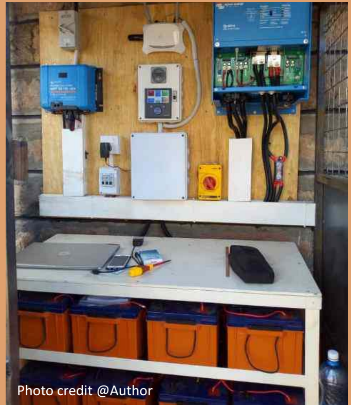
Figure 2: Back-up PV system in a household set up
